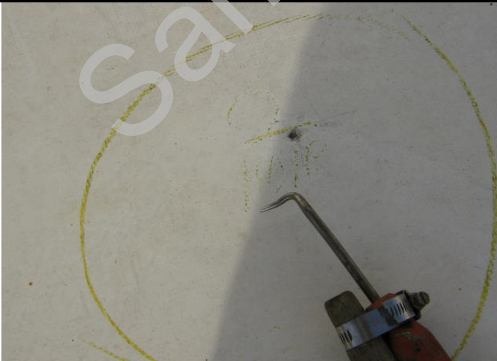
Close up view of one of the three areas of damage. This particular area appears to be a cigarette burn. All three areas were removed as a damaged membrane samples and are included with this report.
