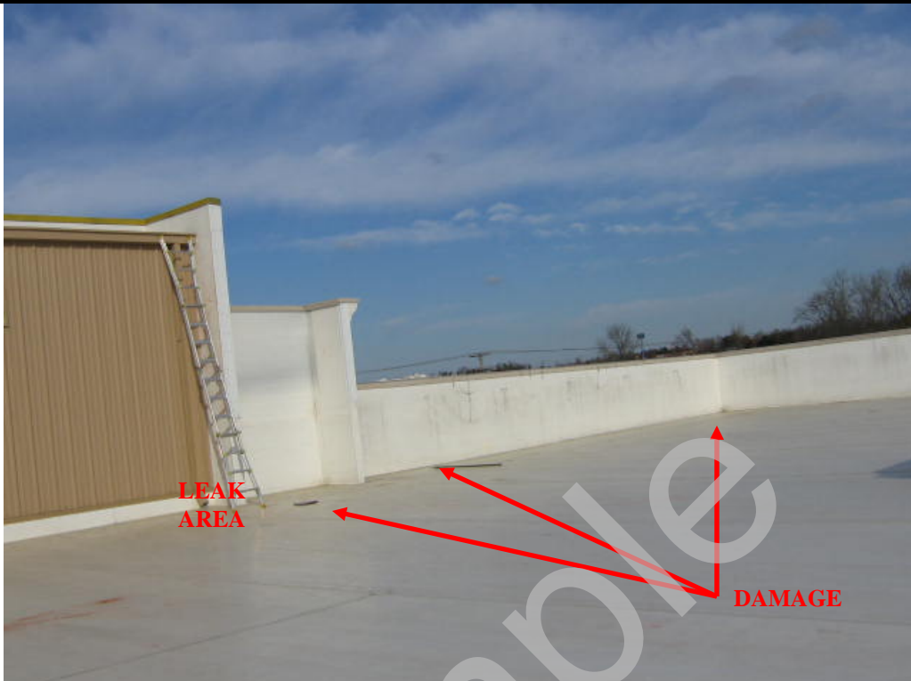
View of leak area as seen from the roof. Roof system was inspected, including the area at top of high wall, and three areas of damage were found in the TPO membrane. Damage was found 5', 15', and 60' from the leak area.
